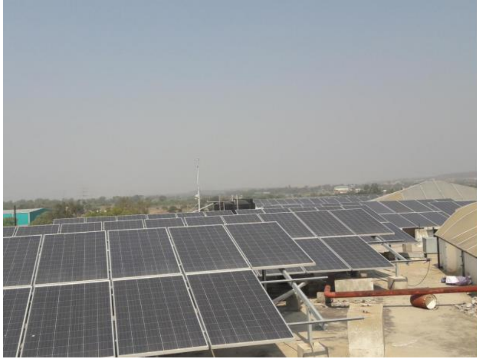
Rooftop Solar Power Plant
